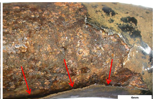
Figure 8. Corrosion progressed along the interface between the coating and the steel, peeling the coating off the spring.
