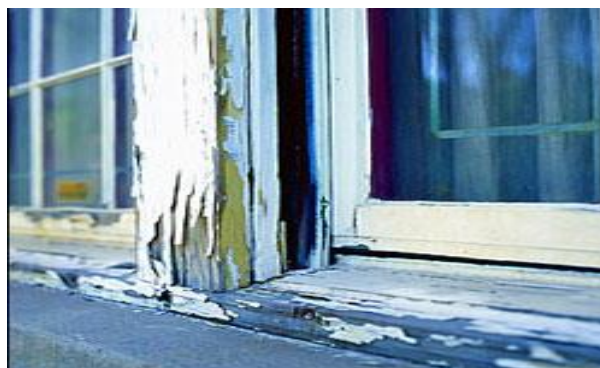
Fig.4. Lead paint peeling as part of a renovation
